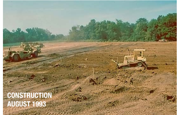
FIGURE 5. Reshaping and adjustment of the wetland floor to designed elevations. “Topsoil” materials were stockpiled and re-applied six to twelve inches deep to approximate the final finished elevations of the wetland floor and to act as the wetland “substrate” (the medium for plant growth and the microbial/invertebrate microbiome).
